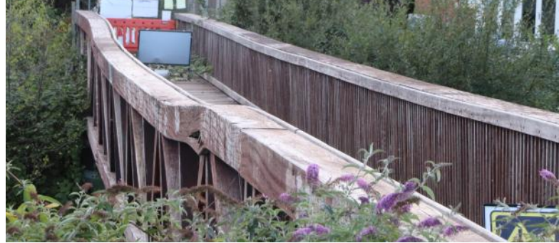
Upper structural member: split and bending
